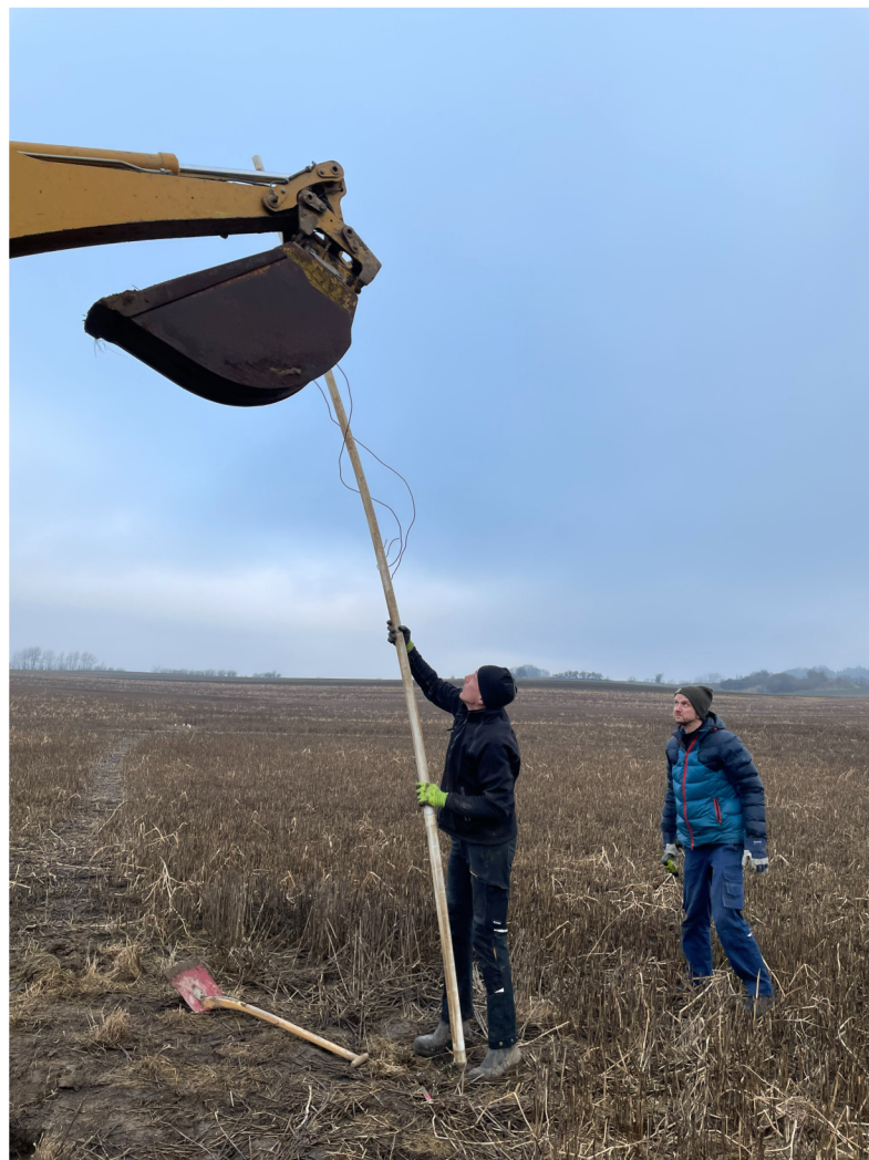
Piezometer installed at two field sites from 0–5 meter. In total 180 piezometer were installed.
